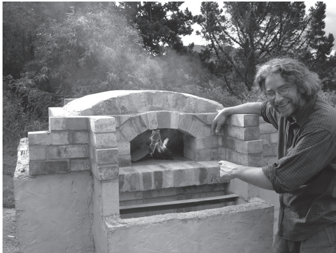
Two studies of David Parker's oven in construction. The upper picture shows the lower blockwork, with the lintels in place to take the sole of the oven itself. The lower photograph shows the oven completed before the chimney and superstructure have been built. (Photographs, David Parker)
